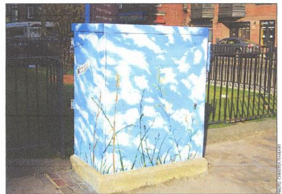
Traffic signal box in the South End painted by Christos Hamawi
